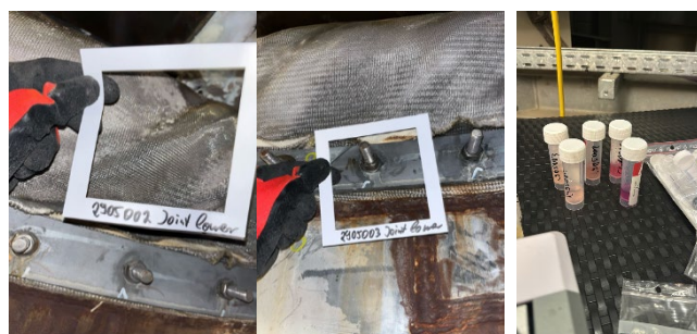
Figs.14&15: Expansion joint of the turbine
