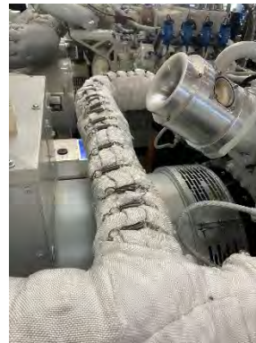
Fig. 66/Fig.67 CHP exhaust pipe insulated calcium-free
