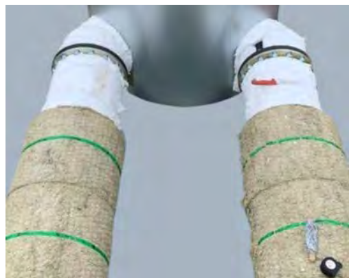
Fig. 81: Industrial insulation with chromate blocker
