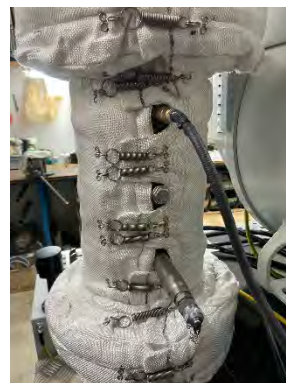
Fig. 68/Fig.69 Exhaust pipe CHP unit insulated calcium-free
