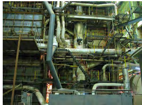
insulationFig. 8: Power station insulation
