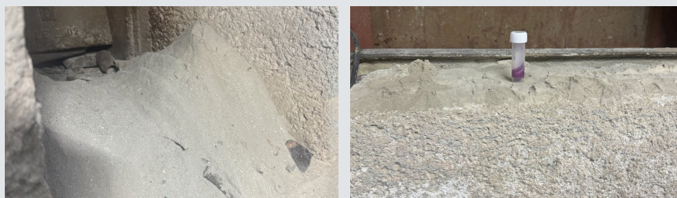
Loose ash layer on a component in the furnace area. Detection in ash in the furnace area, sample tube with colour change.
